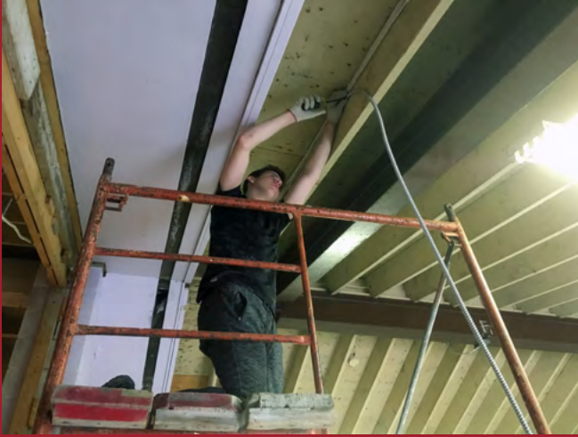
Frederic Litwin helps with electrical installations under the supervision of Mr. Leszek Rudowski. Spring 2018
